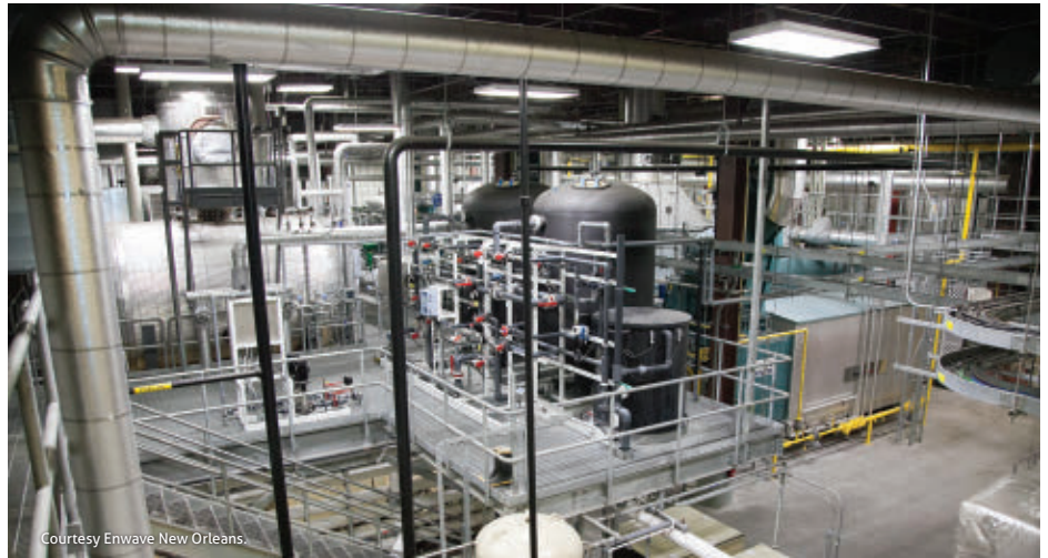
The reverse osmosis system and piping at Enwave New Orleans' steam plant.
